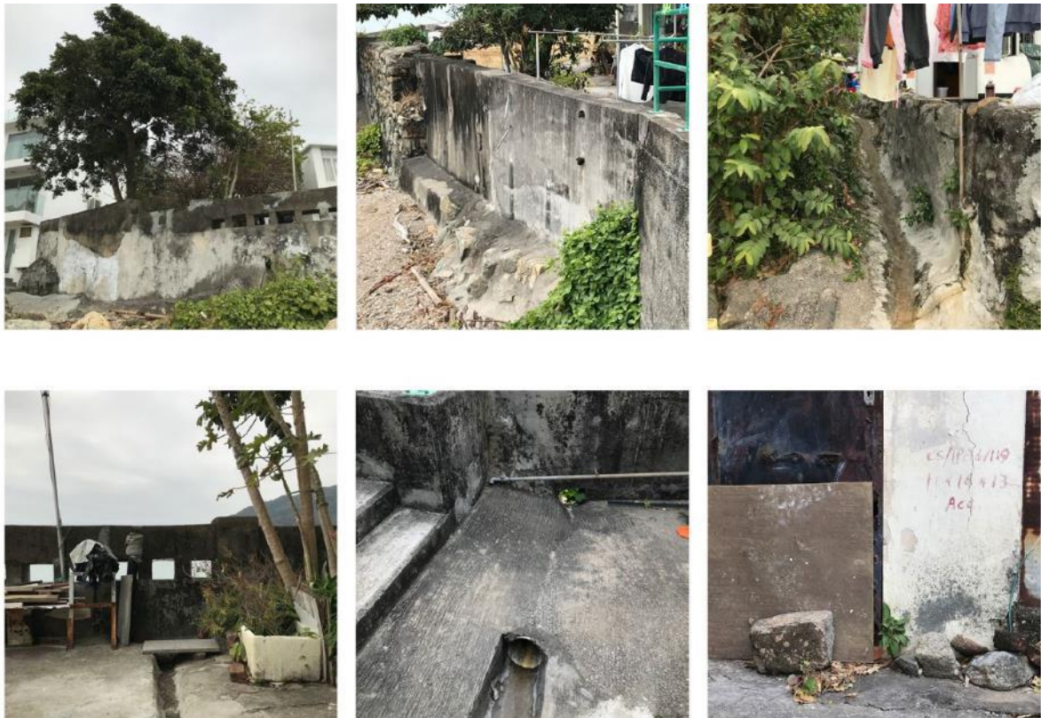
Plate 4.77: Stone embankment along the coast, photo taken by the research team in 2021.
