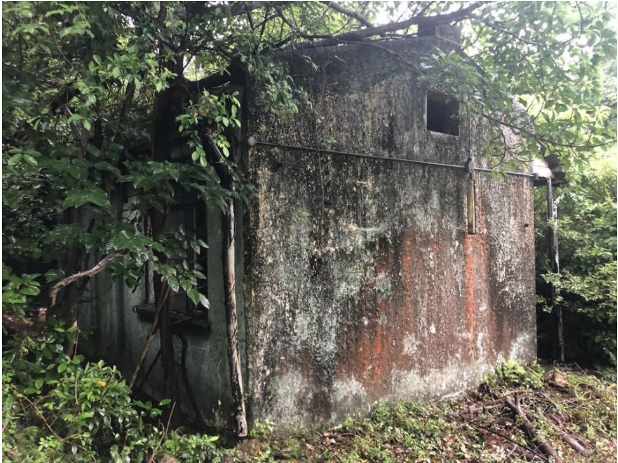
Plate 7.80: No. 11 Shek Pik Reservoir Road, photo taken by the research team in 2021.
