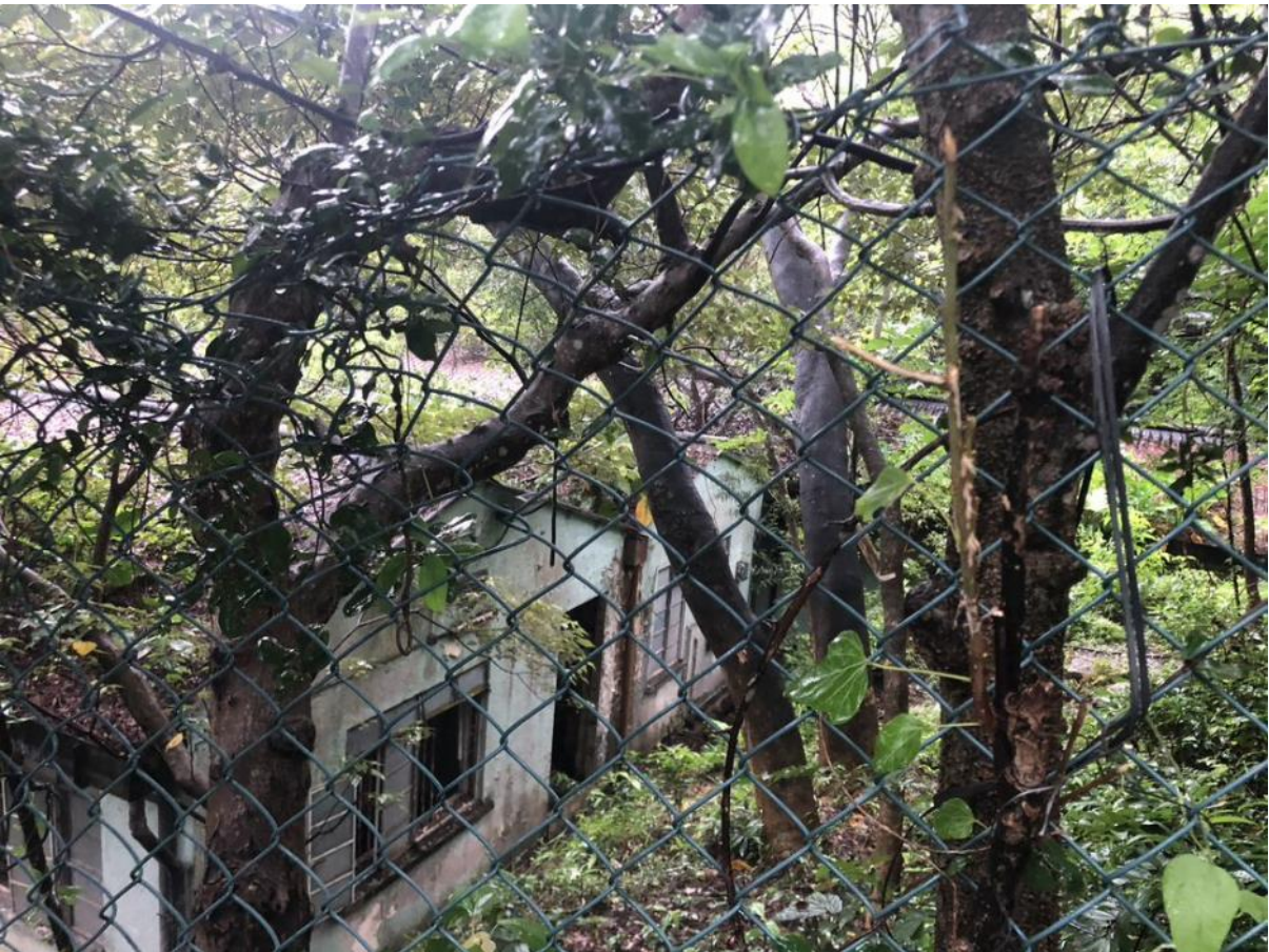
Plate 7.77: No. 3 Shek Pik Reservoir Road, photo taken by the research team in 2021.
