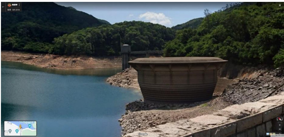
Plate 7.66: Shek Pik Reservoir Bellmouth Overflow in 2018. The ridge of the bellmouth was slightly refurbished 696 .
