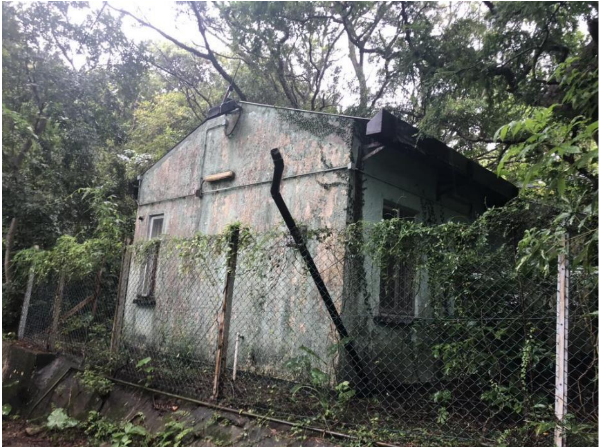
Plate 7.78: No. 4 Shek Pik Reservoir Road, photo taken by the research team in 2021.
