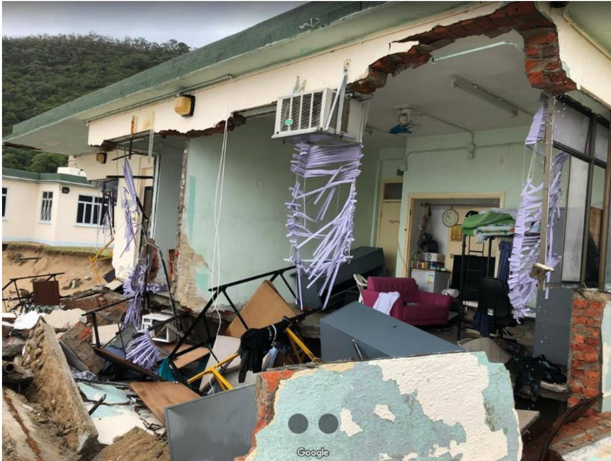
Plate 7.89: The staff dormitory building was severely damaged when Typhoon Mangkhut hit Hong Kong in 2018 734
