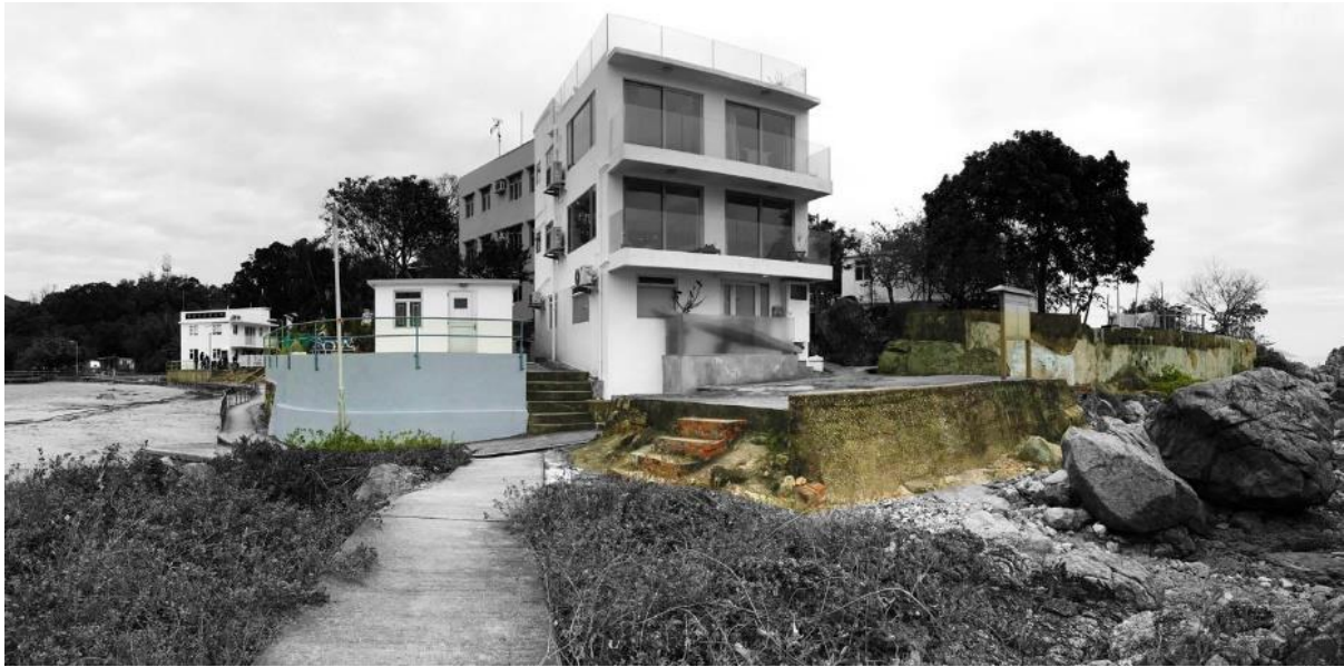
Plate 4.38: Stone embankment along the coast, photo taken by the research team in 2021.
